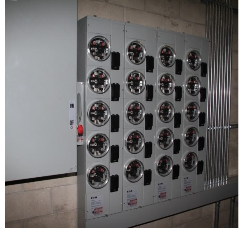
Additional metering capacity for EV charging was added to this high-rise condo community, but most electrical rooms don't have this growing capacity.
