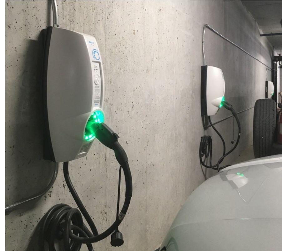
Wall chargers in an apartment parking garage
